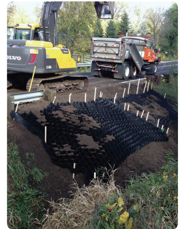
Flooding in 2012 in Northeast Minnesota damaged roads and bridges, water and sewer systems and other infrastructure, costing $108 million. More than 1,700 homes and 100 businesses were damaged or destroyed, costing more than $12 million.
